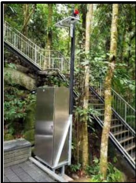
The cabinet at the lower pool, containing the main controller for the warning system.
