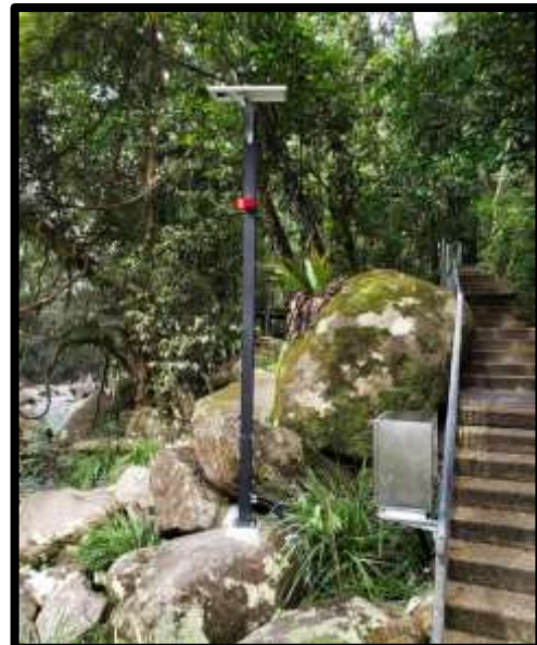
The cabinet at the middle pool, containing the second controller for the warning system.
