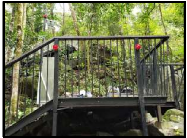
The platform at the lower pool, showing three of the four beacons installed at that location
